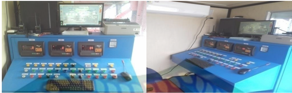
Gambar 5.2. Panel Monitor Batching Plant (Dokumentasi 2020)
