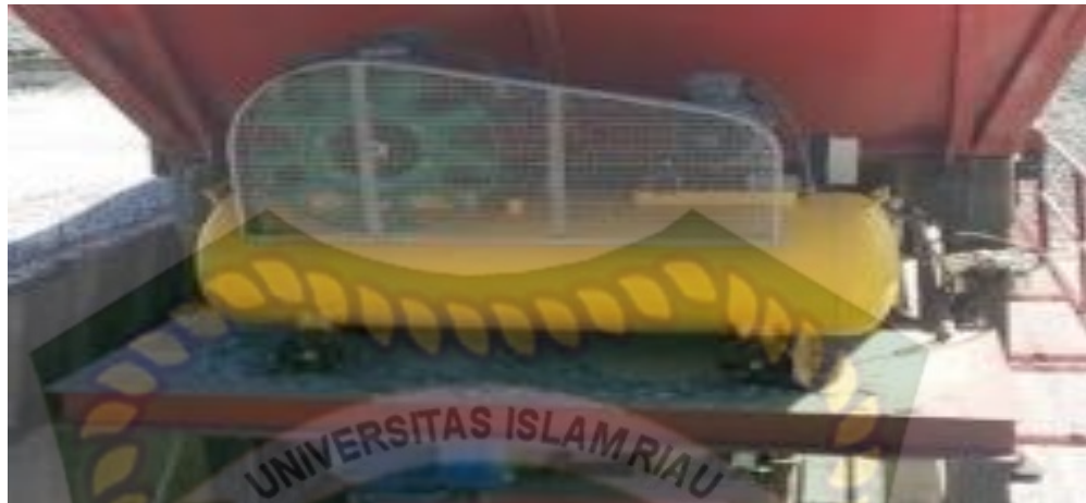
Gambar 5.14. Compressor Batching Plant (Dokumentasi 2020)
