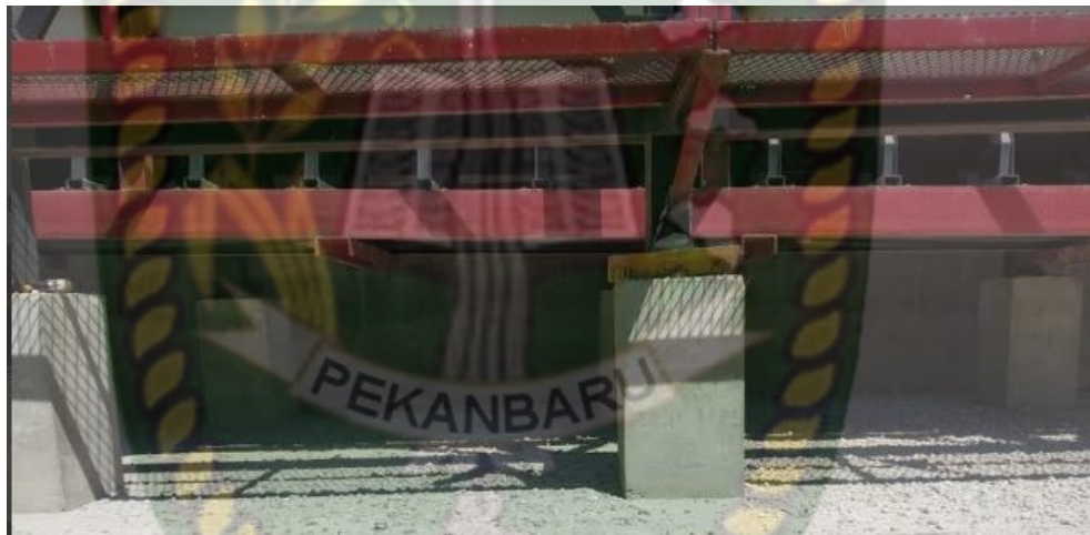
Gambar 5.5. Belt Conveyor Datar Batching Plant (Dokumentasi2020)
