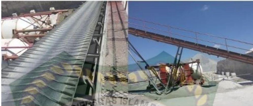
Gambar 5.6. Belt Conveyor Datar Batching Plant (Dokumentasi 2020)
