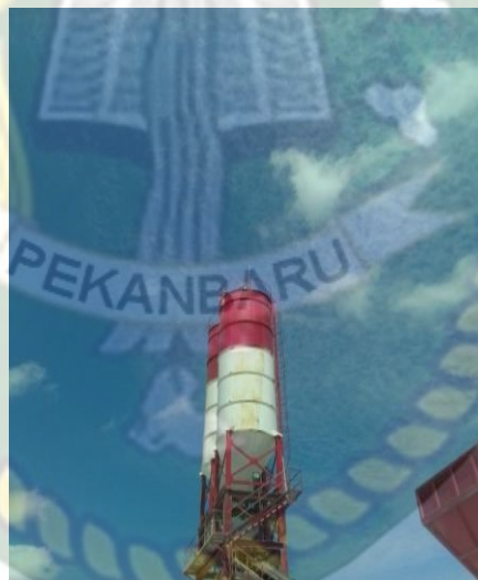
Gambar 5.8. Silo Batching Plant (Dokumentasi 2020)
