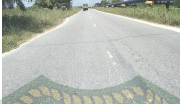
Gambar 3.8 Transversal Crack (Retak Melintang) (Suwandi, 2018)
