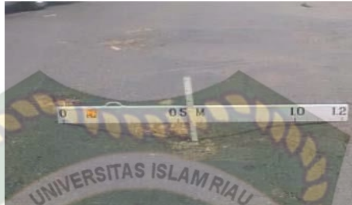
Gambar 3.3 Amblas ( Depression ) (Bina Marga, 1983)
