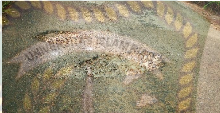
Gambar 3.5 Lubang ( Potholes ) (Suwandi, 2018)
