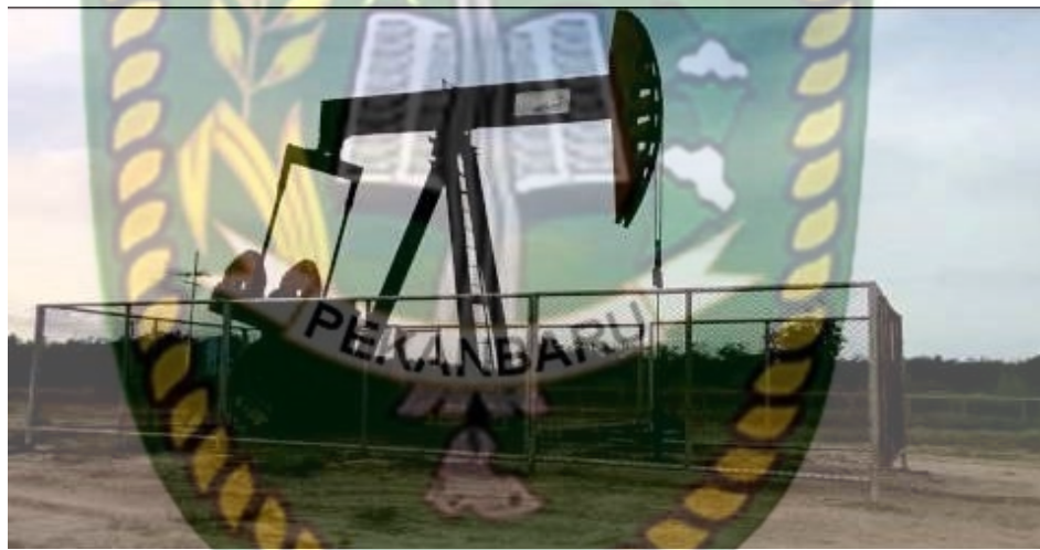
Gambar 4.1 Pompa Sucker Rod Pump
