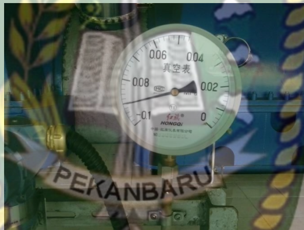
Gambar 3.3 Pressure Gauge (PLTU Tenayan Raya)
