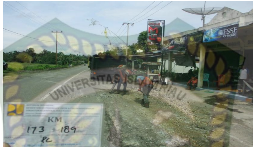
Gambar 14. Galian Perkerasan Beraspal tanpa Cold Milling Machine (Sumber : PT. Hasrat Tata Jaya)
