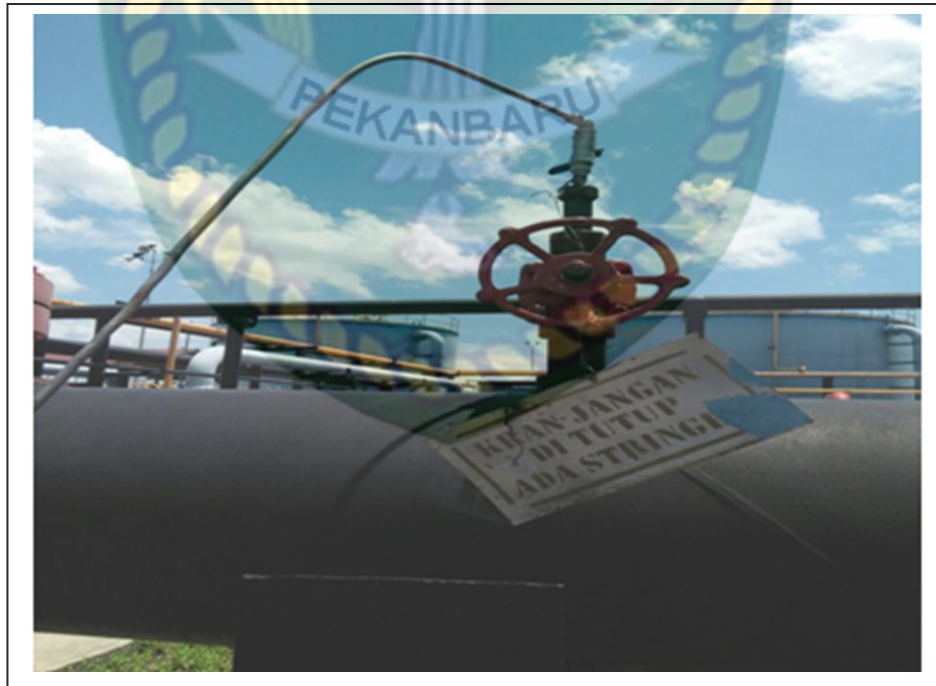
Gambar 2.5. Inlet Injection ke wash tank Biosida
