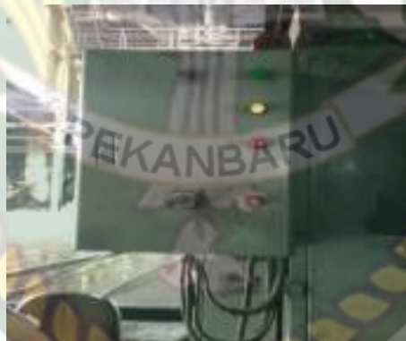
Gambar 3.5 Main Panel (PT. Perkebunan Nusantara V Pks Sei Pagar)
