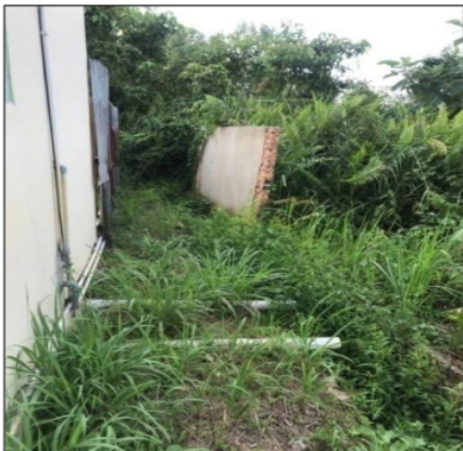
Figure 7. One of the documentation of building damage due to land subsidence
