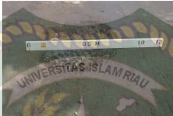
Gambar 3.21 Lubang ( Pothole ) (Bina marga no.03/MN/B/1983)
