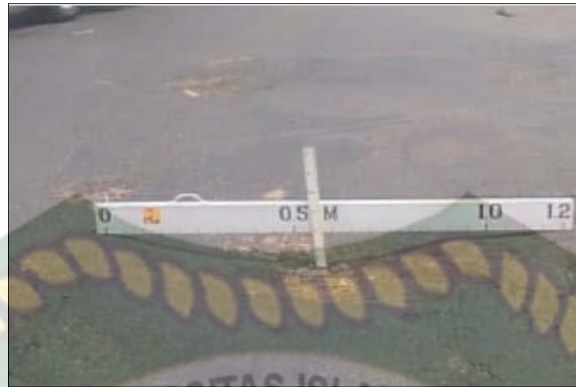
Gambar 3.4 Amblas ( Depression ) (Bina marga no.03/MN/B/1983)
