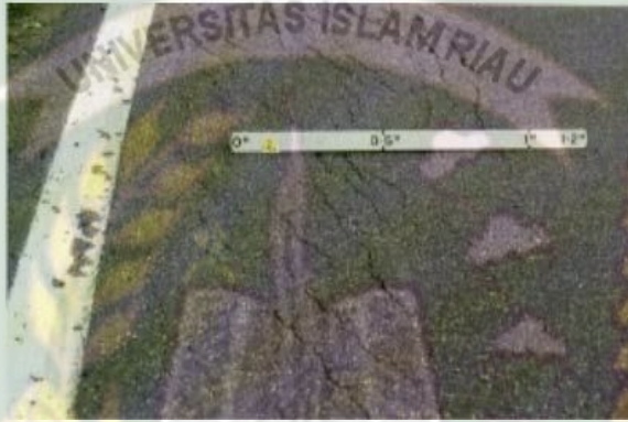
Gambar 3.14 Retak Selip ( Slippage Cracking ) (Bina marga no.03/MN/B/1983)
