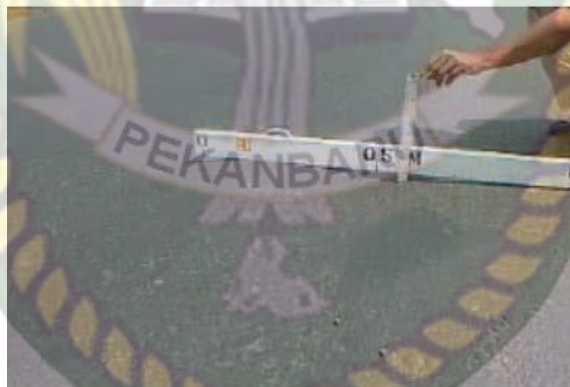
Gambar 3.3 Alur ( Rutting ) (Bina marga no.03/MN/B/1983)
