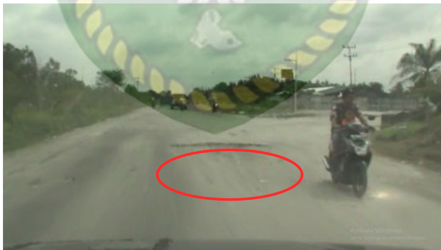
Gambar 5.3 Lubang ( Potholes ) Sta.8+300 (Survei,2018)
