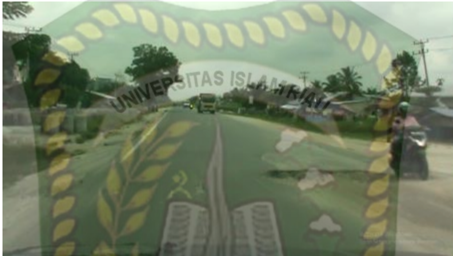
Gambar 5.4 Alligator Cracking dan Potholes Sta.1+500 (Survei,2018)
