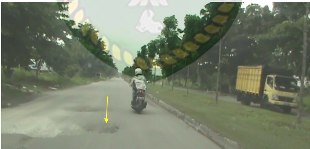
Gambar 5.5 Lubang ( Pothole ) Sta.003+800
