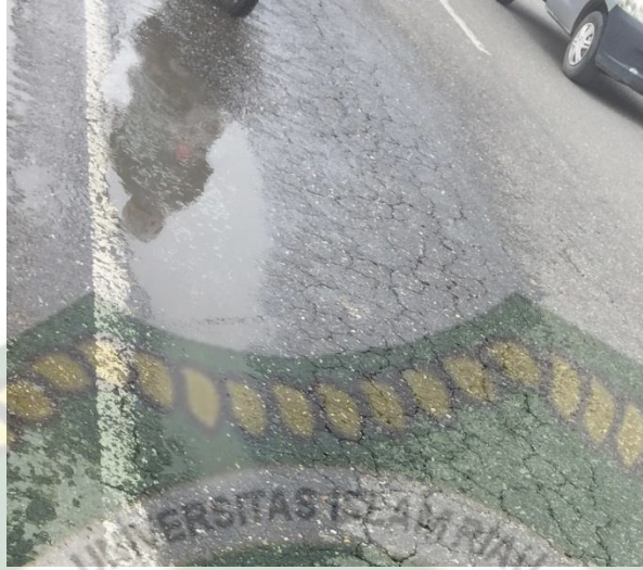
Gambar 3.4 Alligator cracking (Sumber : tosimasipil.blogspot.com,2018)
