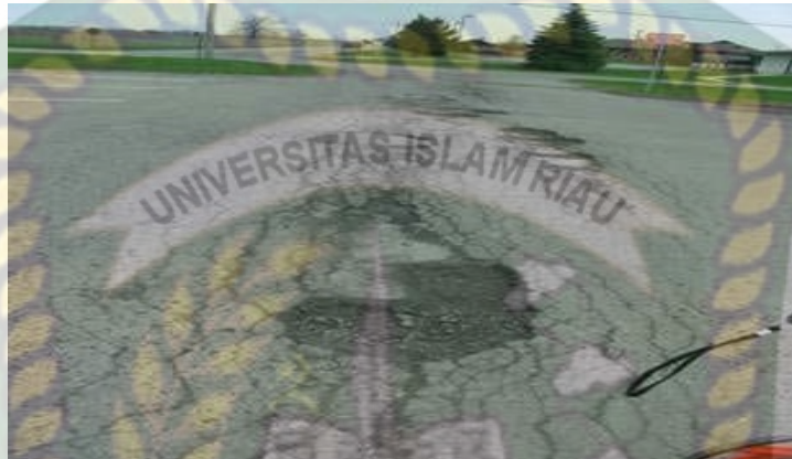
Gambar 3.10 Lubang ( Pothole ) (Sumber : tosimasipil.blogspot.com , 2018)
