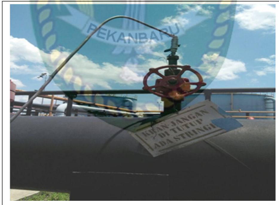
Gambar 2.5. Inlet Injection ke wash tank Biosida
