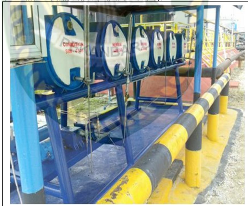
Gambar 2.3. Chemical Pump (Chevron)
