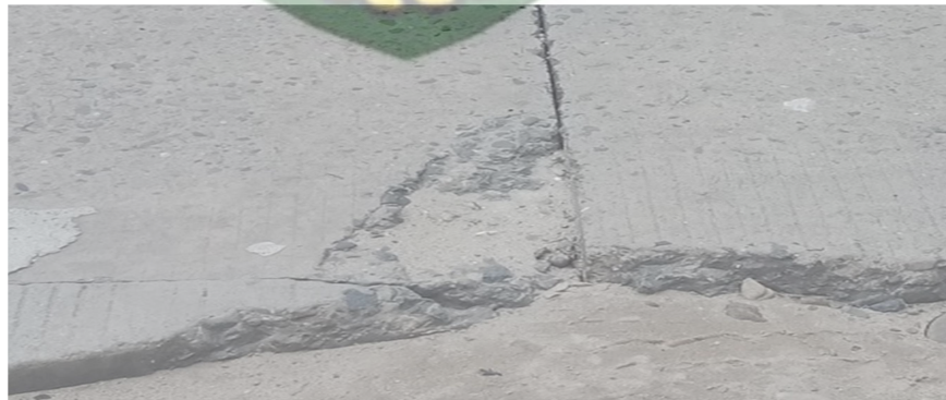
Gambar 3.17 Gompal ( Spalling ) (Survei Lapangan)
