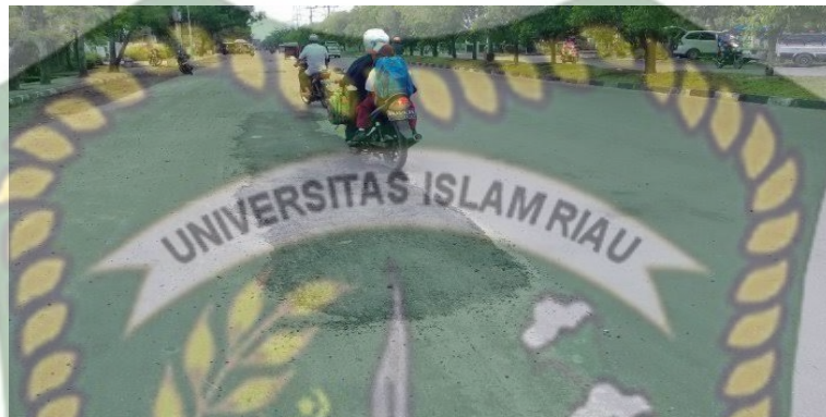
Gambar 3.19 Tambalan ( Patching ) (Bina marga, 1995)
