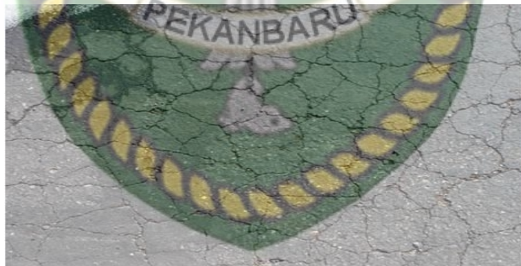
Gambar 3.2 Retak Kulit Buaya (Alligator Cracking) (Suwandi, 2018)
