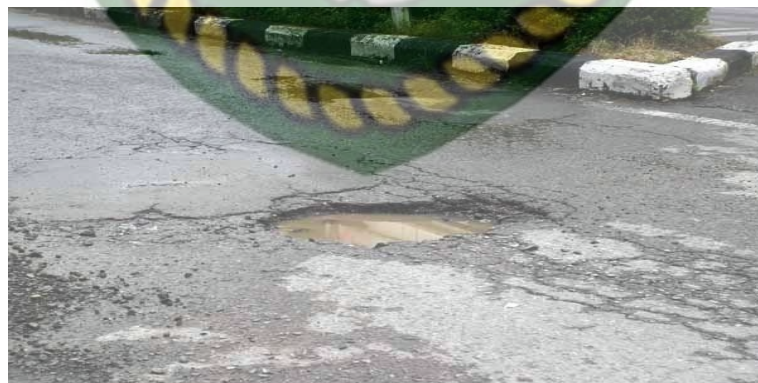
Gambar 3.18 Lubang-lubang ( Potholes ) (Bina marga, 1995)
