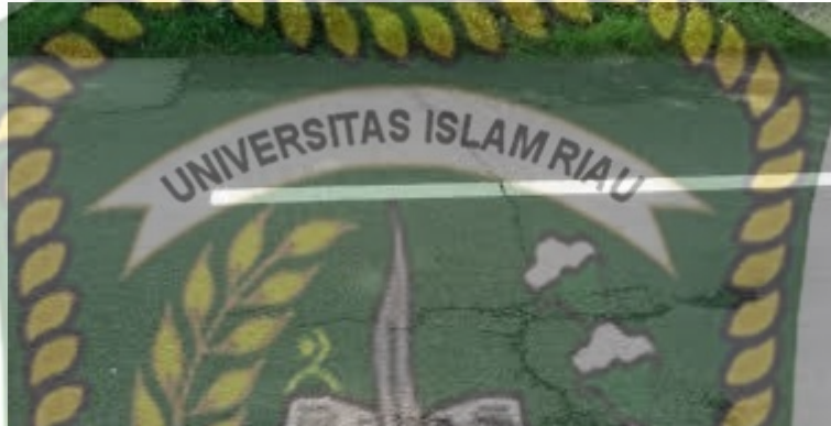
Gambar 3.4 retak blok ( block cracking ) (Suwandi, 2018)
