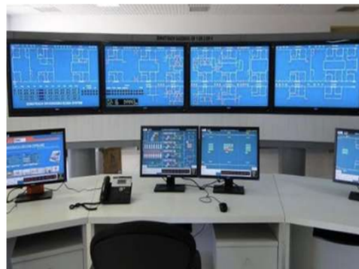
FIGURE 12. Example of control center operation for O&G industry [241].
