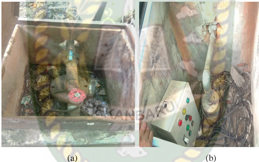
Gambar 5.5 (a) dan (b) Sumur Air Tanah/Deep Well RSUD Arifin Achmad
