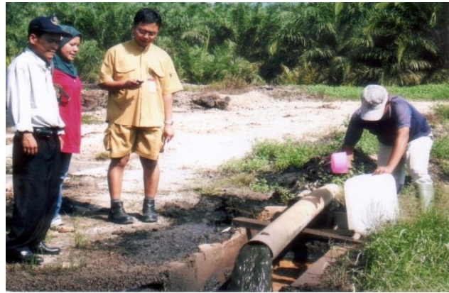
Fig. 6. Waste of CPO in pipe was flowed to sedimentation reservoir throw to gutter.
