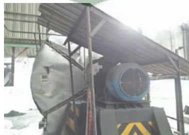
Gambar 2.17 Induced Draft Fan (IDF).
