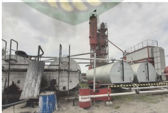
Gambar 3.12 Asphalt Tank (dokumentasi,2019)
