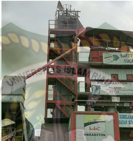
Gambar 3.8 Hot Elevator (dokumentasi,2019)
