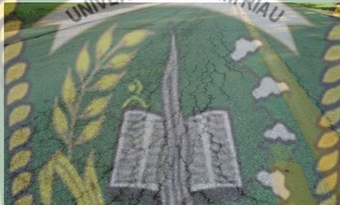
Gambar 3.7 Retak-retak ( Cracking ) ( https://jualbatusplit.wordpress.com/tag/retak-jalan/ )
