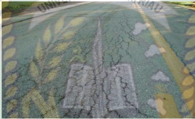
Gambar 3.7 Retak-retak ( Cracking ) ( https://jualbatusplit.wordpress.com/tag/retak-jalan/ )
