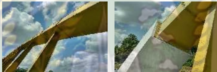
Gambar 5.2 Kondisi Arch Beam .
