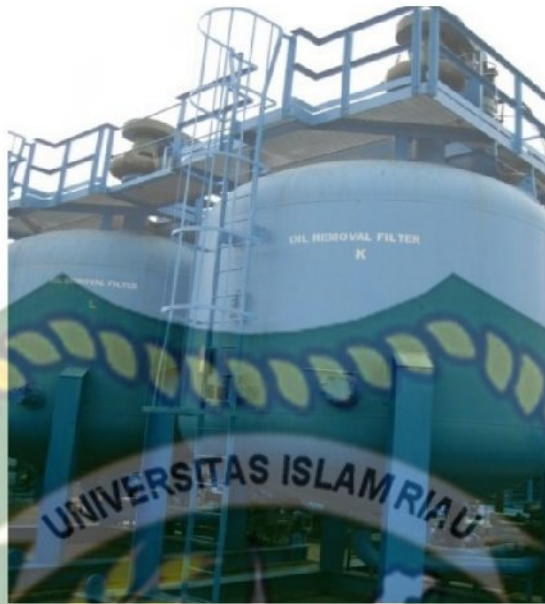
Gambar 2.12 Oil Removal Filter Vertical (sumber data lapangan)
