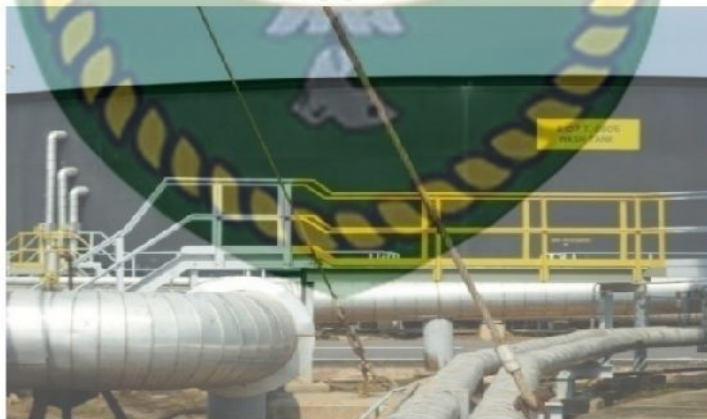
Gambar 2.8 Wash Tank (sumber data lapangan)
