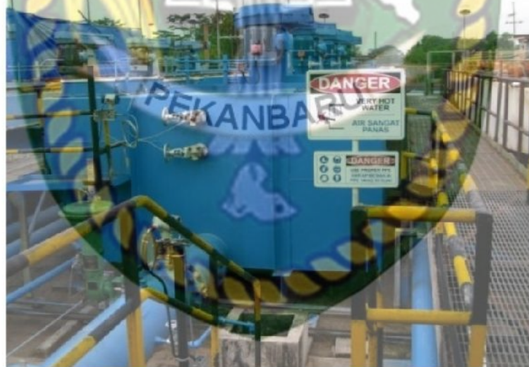
Gambar 2.10 Mechanical Floatation Unit (sumber data lapangan)
